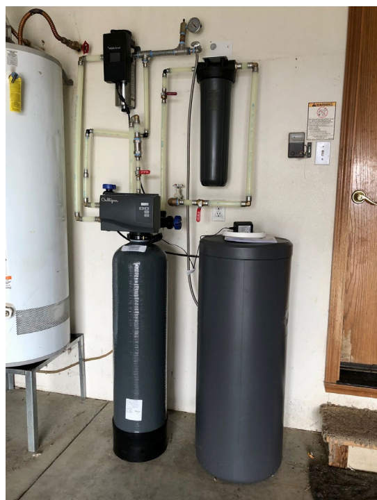
Installed whole-house treatment system
